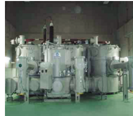
SF 6 Gas Transformer
